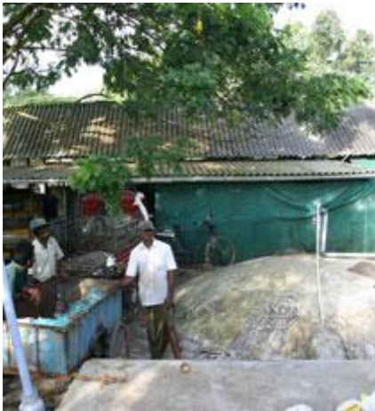
A biogas plant in Cochin, Kerala.
